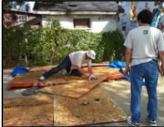
David Espinosa and Edgar Kusnohadi hard at work cutting wood for the roofer.
